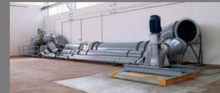
Sala prove Testing Room
