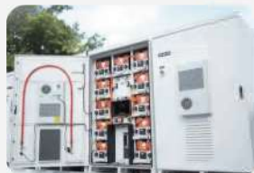
Energy storage container
